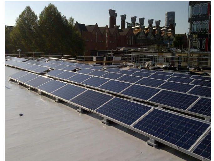
De Montfort University Leicester/ UK 49,92 kWp (2015)
